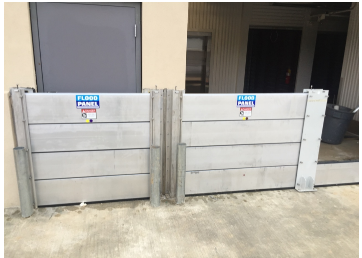
Flood Panels - Installed
